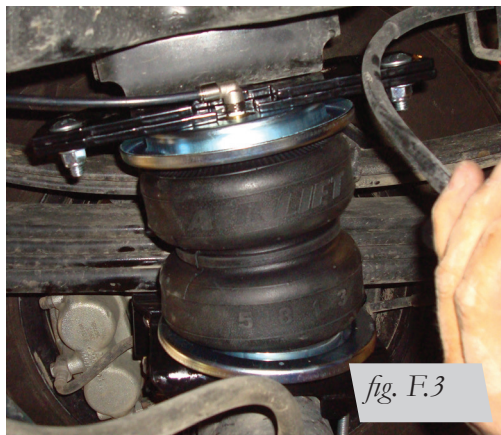
Inside view of the driver's side installation.
